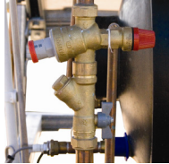
Figure 3.15 Pressure Control Valve
